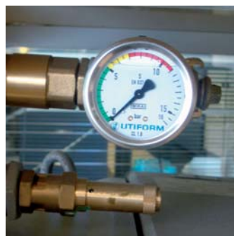
Air pressure meter and safety valve
